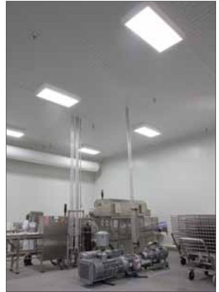
Kenall’s SimpleSeal provides safe lighting for U.S. Pet Nutrition plant in Lyons, GA
